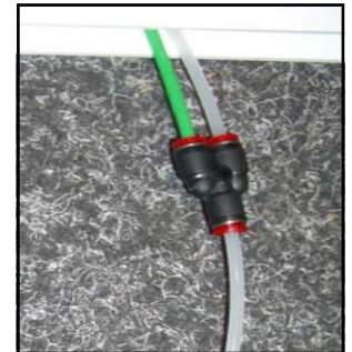
Bleed kit Y piece connected to pipes protruding from underneath skeg box
