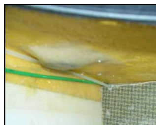
Example of tube routing through bulkhead immediately below deck
